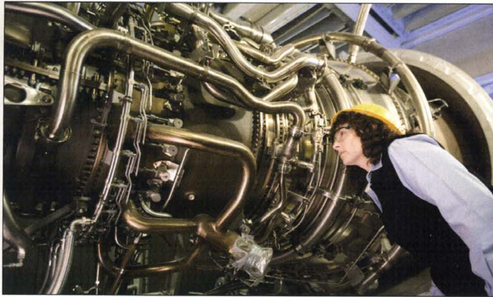
Public Relations Analyst Dianne Porter gets a close up look at the LM6000 combustion turbine at the North Pole Expansion Plant. Plant construction is expected to be complete this fall.
