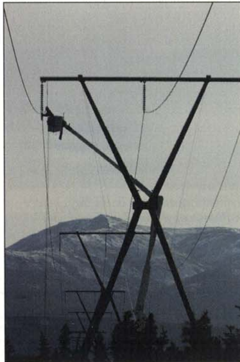
The Northern Intertie has prevented outages due to the reliability created by separate routes for the two interties from Healy. Most recently during the forest fire in Nenana which necessitated deenergizing one of the transmission lines for firefighting safety.
