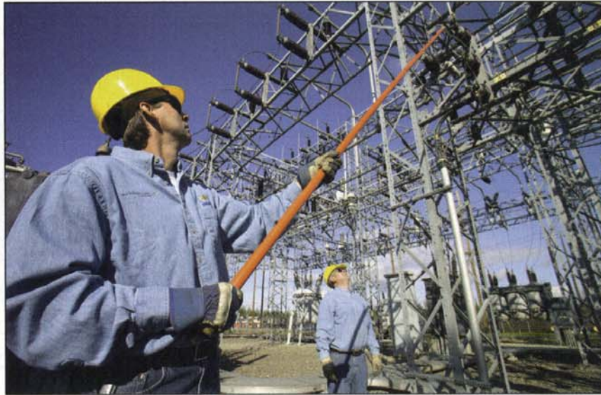
Linemen Frank Stoneman and Walt Becker operate a by-pass switch at one of GVEA's 35 substations.
